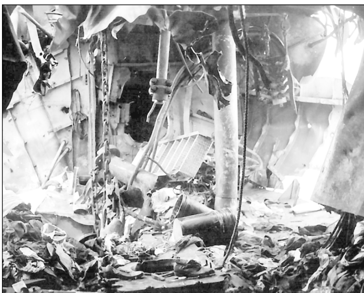
TWISTED METAL -- This photo taken from the inside of the Rodman's hull shows the extent of damage caused by the first plane to strike.
